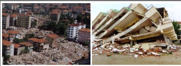
Figure 2 Building damage in Golcuk (courtesy of R. Andrews)
